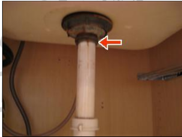
4.0 Picture 1 Right sink basin
