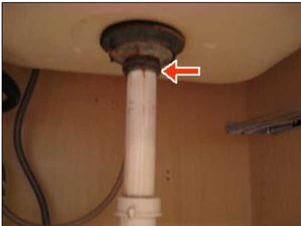
4.0 Picture 1 Right sink basin
